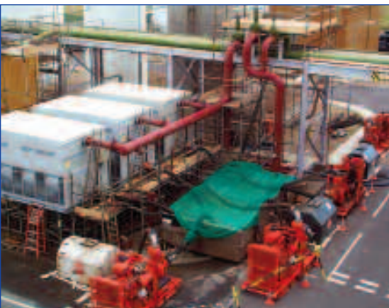
North East Chemical Processing Plant. Carrier Rental Systems provided a package of 3 x 2000kW cooling towers and 3 x high head circulation pumps during a planned maintenance period.
