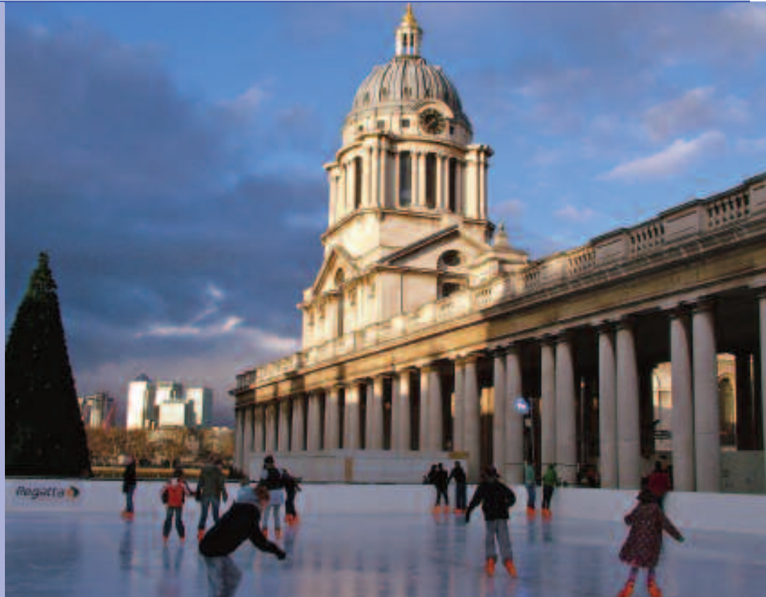
Greenwich Ice Rink 08. Carrier Rental Systems provided a complete package of 3 x 450kW chillers, 2 x 500 kVA silenced generators plus ancillary equipment
